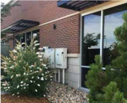
Utilities screened on the side of the building
